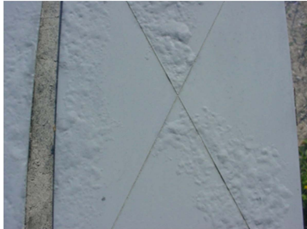
Corrosion Mechanism in Outdoor Exposure Testing
